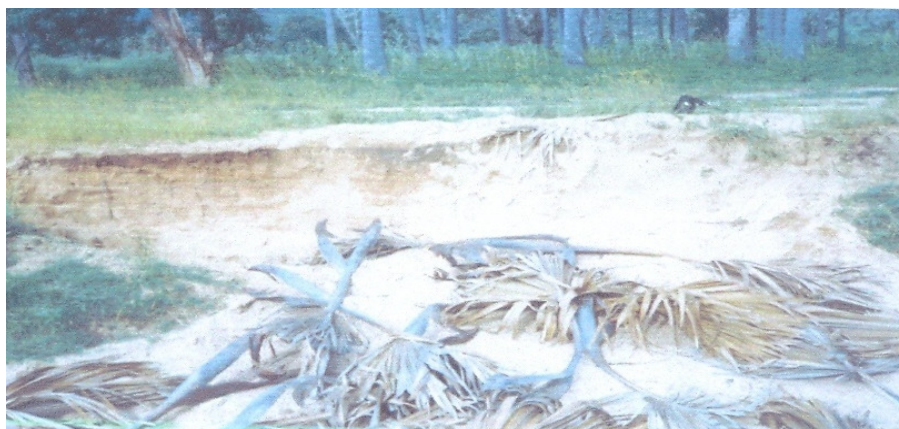
Plate 2: Showing Gully erosion cutting across a road in Lum
